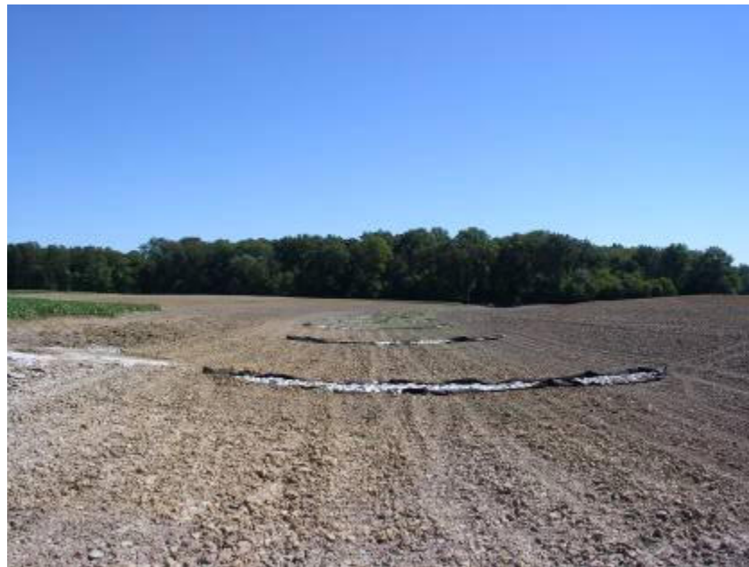
Rock checks installed to reduce runoff velocity in a waterway in St. Clair County, Illinois (Office photo StC1000)
